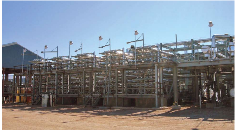
ABOVE: EOR CO 2 recovery plant (89% CO 2 ) using Grace CA spiral wound membranes. Zero hydrocarbon losses – 100% of permeate gas stream being compressed and reinjected (> 95% CO 2 ). APPLICATION: EOR CO 2 Gas Recovery.
